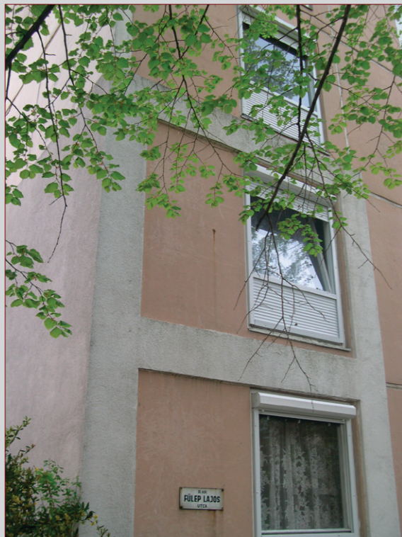
At the joint of the panels the material of the weather strips shrank and created ways for the cold to infiltrate.
