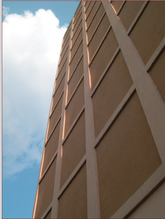
POST-INSULATION TENDENCIES when the lack of governmental subsidies and the nature force the occupants to act on their own...
